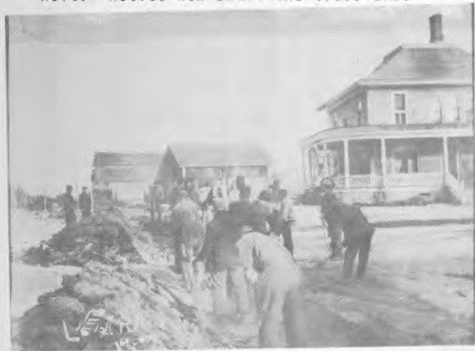
Getting ready to lay the tracks for a rail- road track across East Delhi Avenue in Holt. Notice how small the trees are.
